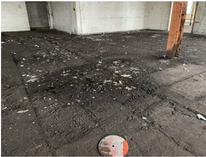
Photograph 1 Undercoat Material on Ground Floor)
