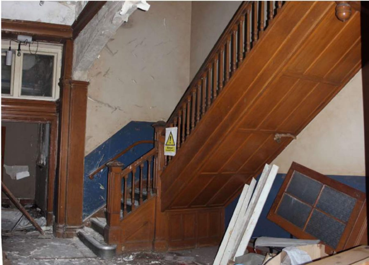
Figure 3: View of the timber staircase and balustrade to the main staircase in Room G.26 of Factory No. 2.
