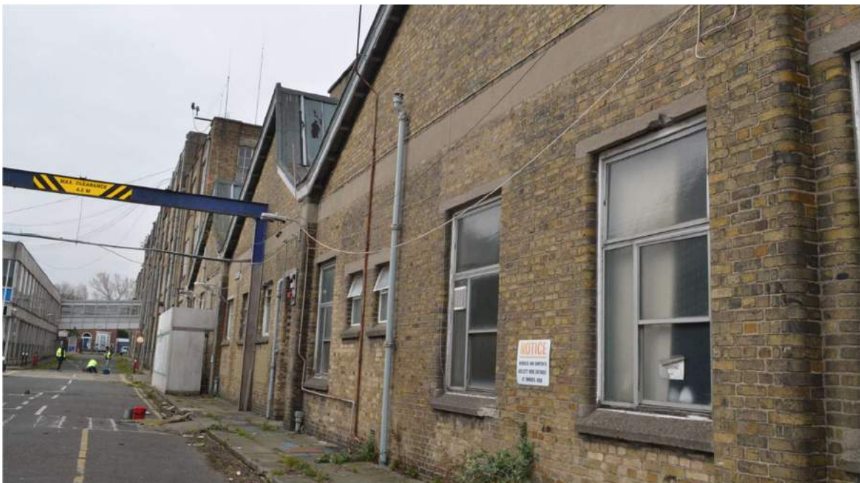
Figure 1: View of the historic brickwork to Factory No. 1, to be demolished as part of the proposed redevelopment.
