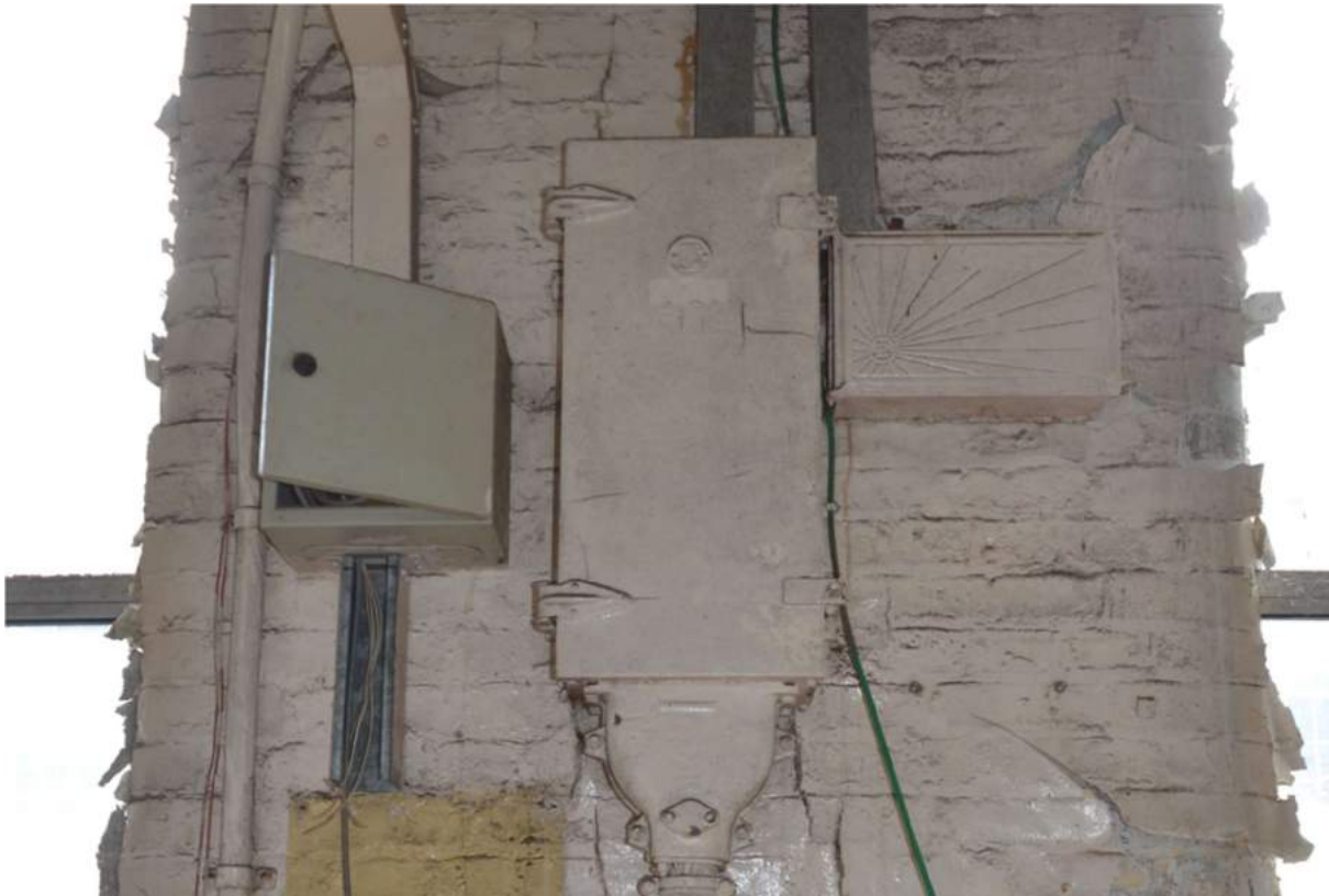
Figure 10: Decorative cast-metal cover to services box.
